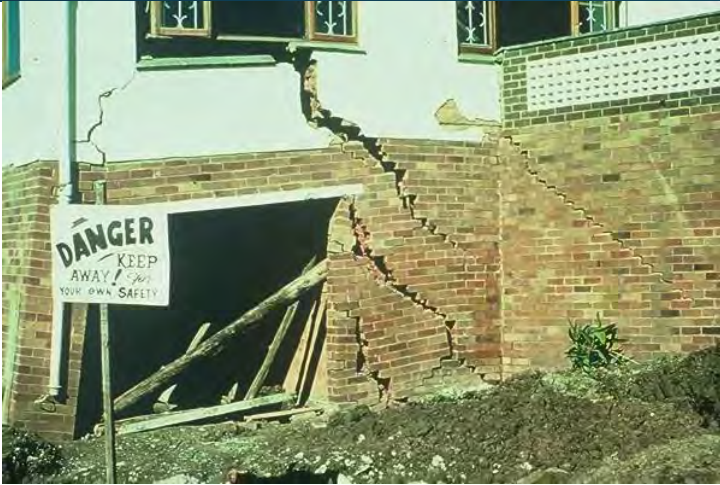
Damage due to heaving clays
