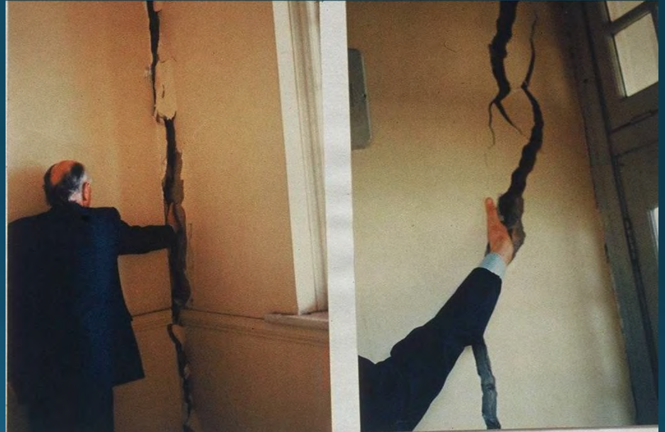
Damage due to collapsing sand
